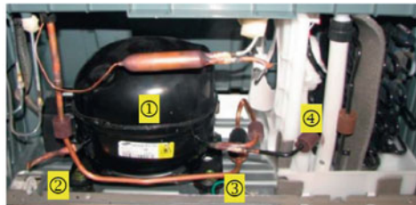
(b) Machine compartment: (1) compressor, (2) rubber, (3) connecting tubes, and (4) fan and condenser
