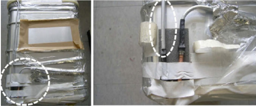
(a) Pitted evaporator tube in field
